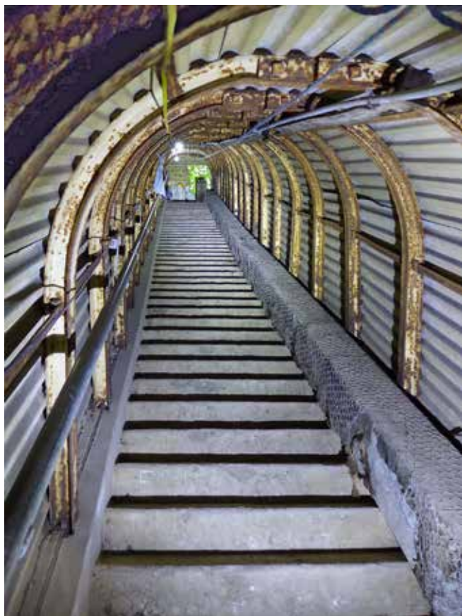
Fan Bay entrance stairs; until the entrance by the sound mirror was reopened, this was the only way into the shelter. Original ventilation trunking is still in place. Photo Tim Wellburn
